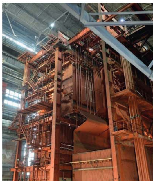
Figure 1. Metal frame with suspended equipment (steam boiler)
